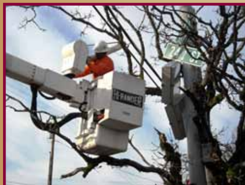
Crews work to repair a traffic signal after a large Oak tree fell on it.
