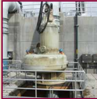
Pulling influent pump for inspection and maintenance.
