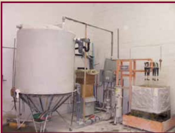
Typical pretreatment setup inside a small permitted industry.
