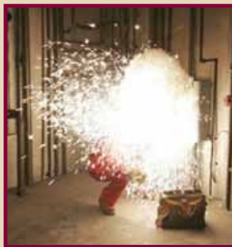
This photo is an example of an arc flash.
