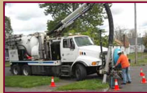
Using a Vac truck to remove debris from a stormwater catch basin.
