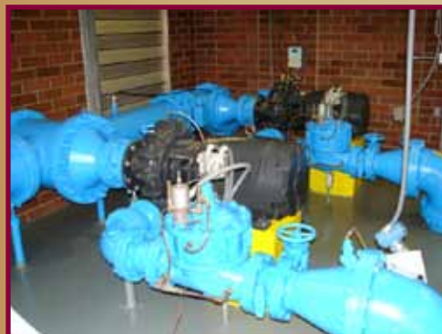
Deer Park Water Pump Station.
