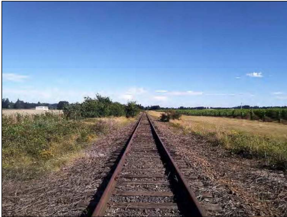
Figure 63. Overview of TS02, facing northwest from its intersection with Jordan Road SE at the southwestern extent of the proposed acquisition parcel.
